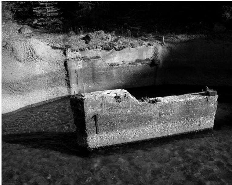
Damage to the EID Canal west of Kyburz
